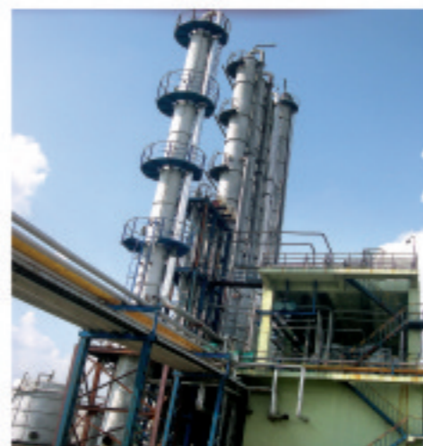
炼油蒸馏装置 Refining and distilling equipment
