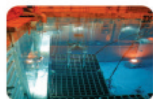
核反应水池 Nuclear reaction water tank
