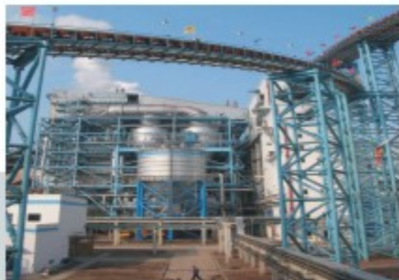
■ 电站锅炉 Power Station Boiler
